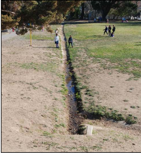
Exposed drain swale - Replace with new storm drain line
