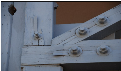
Concern with exterior dry rot
