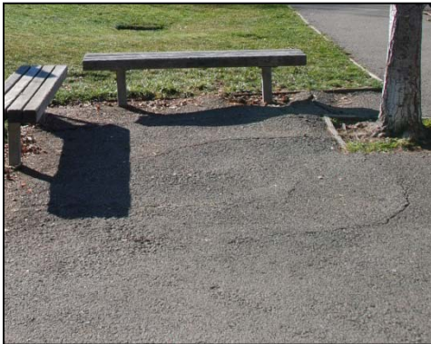
Some paved areas in need of repair
