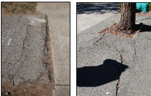
Numerous areas of poor paving and accessibility issues
