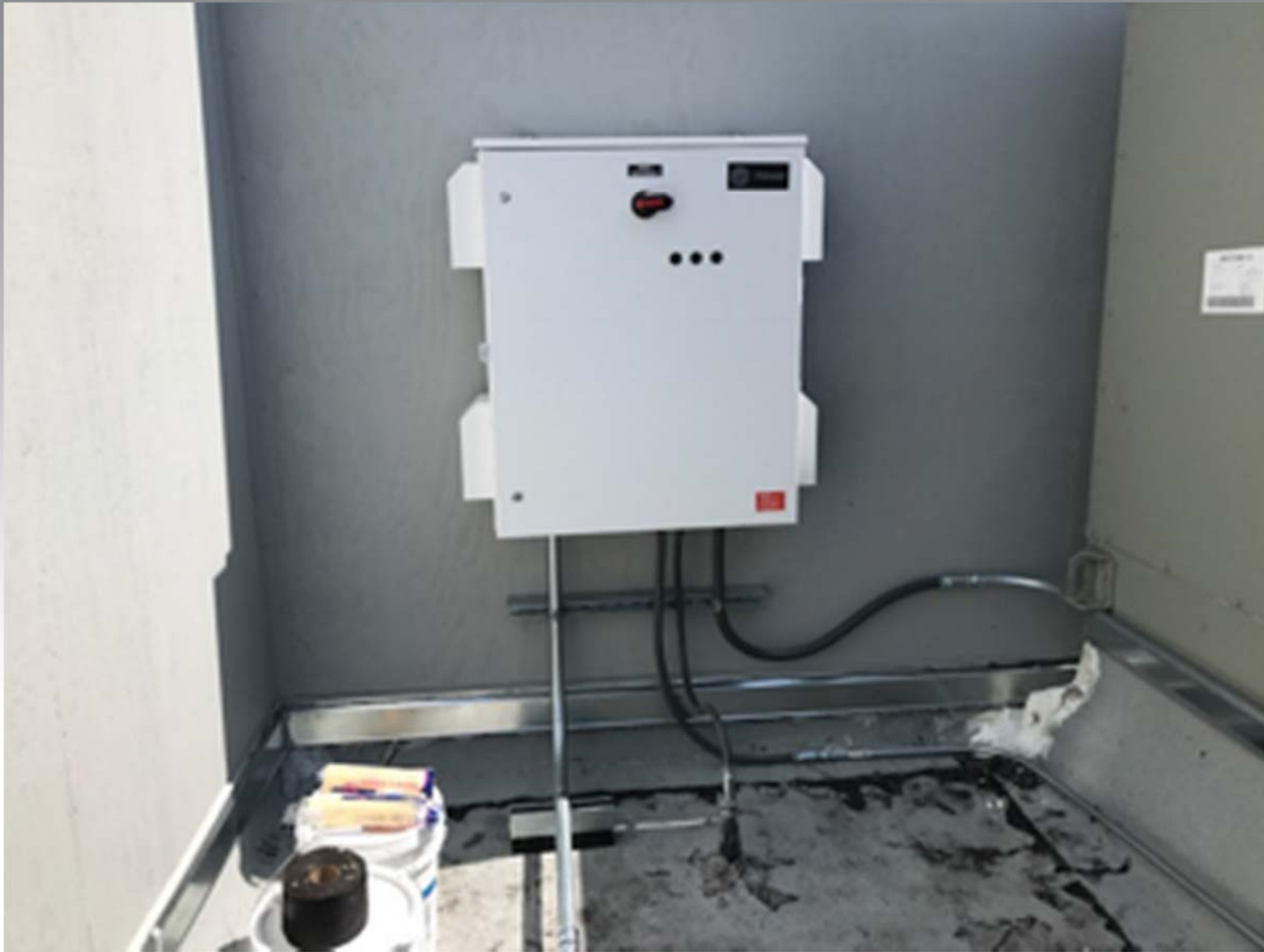
AHU-1 Electrical and controls panel installed
